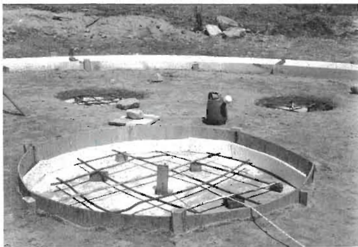
Fig. 3.21: Formed with \frac{1}{4} " plywood, the footing for the masonry stove is ready to pour.
