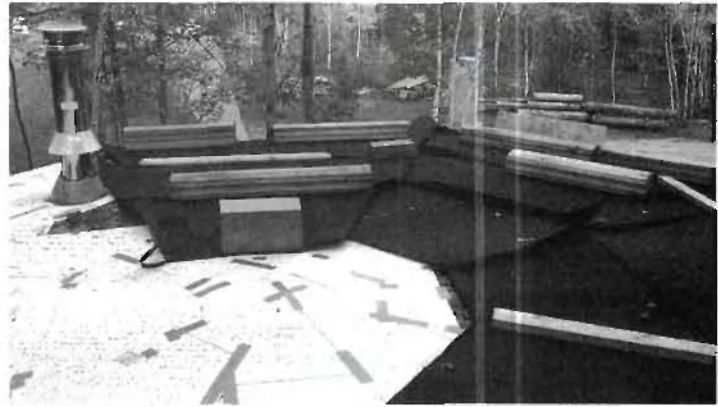
Fig. 8.7 (left): Installing a woodstove chimney. Any projection cut through the membrane has to be treated very carefully, with both waterproofing and drainage. As our Metalbestos® stovepipe has an 8" outside diameter, we made a hole of 12" in diameter through the Bituthene®-covered planking. A reciprocating saw works well for cutting the hole. This way, the chimney has the required 2" clearance from combustible material. The Roof Support Package (Metalbestos® part RSP) unit shown has two adjustable metal flanges which can be screwed to the planking, allowing the installer to plumb the stovepipe itself to a true vertical.
