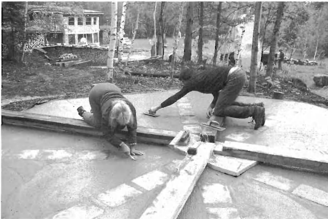
Fig. 10.4: Jaki points around slates set into the fresh concrete at Stoneview, while intern Nick Brown hand-trowels the triangular spaces between the eight slate "spokes."
