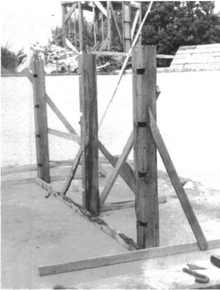
Fig. 6.4: We temporarily braced the support posts for the main girders. nicely by itself, take it down and measure and mark the other end. You only get one try at the top end, so be careful. On the plus side, if it is a little off, the error can always be made up with wooden shingles.
