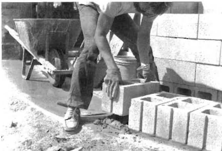
Fig. 5.10: The prudent course of action is to have your wall plans checked by a structural engineer, who can advise you on the need and placement of bond-beam courses and filling cores for bearing pillars. Earthwood: the first course of 8" corner blocks is set in mortar.
