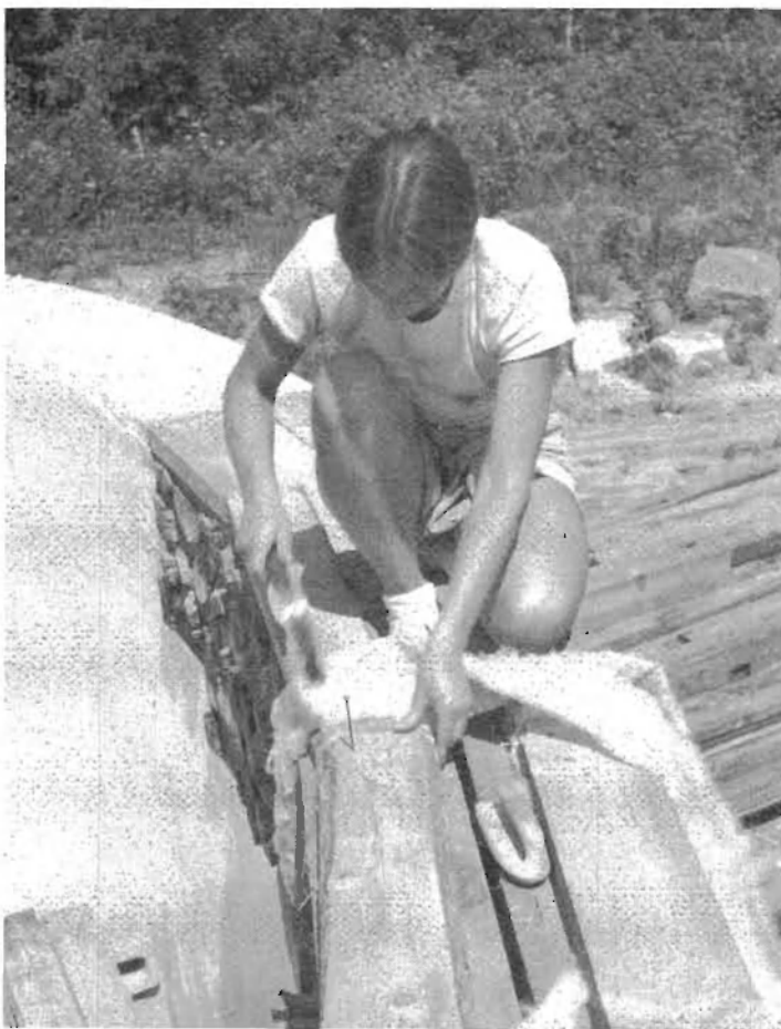
Fig. 6.16: Jaki fastens the wooden plates to the four-by-eight window lintels with 16-penny (3¼-inch) nails. To stop draft, she has installed a strip of fiberglass insulation between the plates and the lintels.
