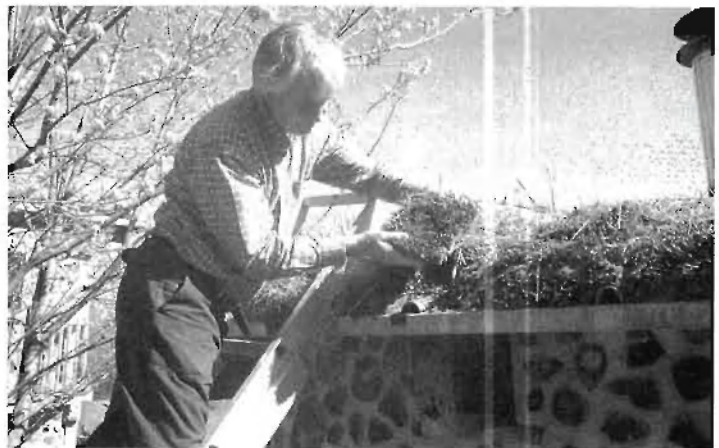
Fig. 8.16: The author installs a moss sod on the edge of the office roof.
