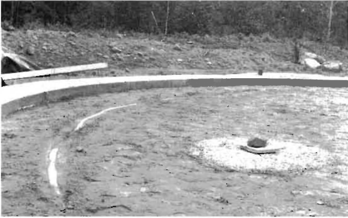
Fig. 4.4: did a good job of spreading and “backblading” 4” perforated the sand to a consistent four-inch depth. The next drain tubing is day, we hired a power compactor to tamp the set into the sand. Jaki watered the sand with a watering can – sand pad. we had no running water on site – while I ran the machine. Hitting each square foot three times with the compactor results in a solid base for the concrete floor.
