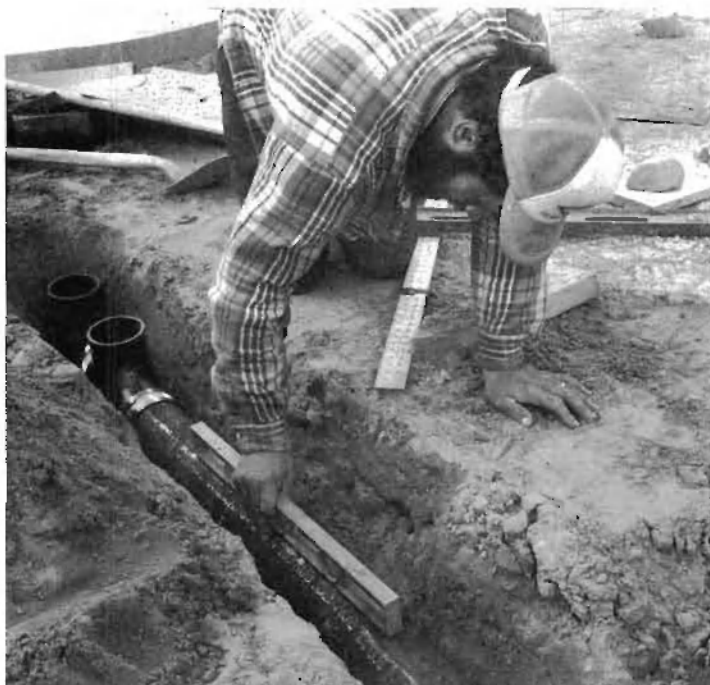
Fig. 4.10: Installation Tips for Underfloor Plumbing Dennis Lee checks the slope of the underfloor drains. Plan the plumbing so that all traps are accessible. In the case of a bathtub or shower on the first floor, this will usually necessitate “boxing out” a small area so that concrete cannot get in around the trap or drain. An 18-inch square box made of 2-by-6 material can be seen in Figure 4.9. It provides access to our shower drain and trap. Another good reason for the box is that – thanks to the ubiquitous Mr. Murphy of the famous law – it is very difficult to get the drain in exactly the right place with respect to adjacent walls, which are still non-existent at this point in time. Within the box, you can still make final adjustments to a drain location at the time of shower- or tub-base installation.
